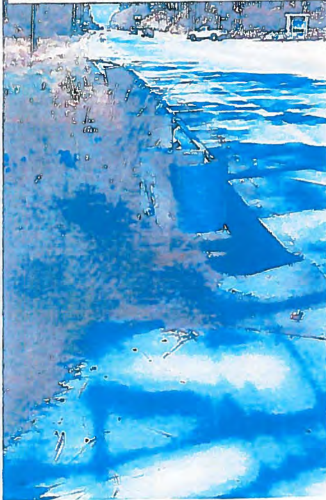
Picture 5: East side of Alf Coleman Road looking south. Guardrail near Harrison Walk Subdivision where storm pipes are to be extended and new headwall constructed.
