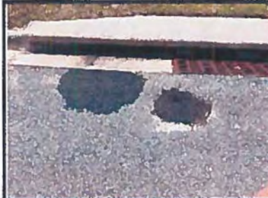
1. Photograph depicting two (2) patches observed adjacent to a drainage inlet in the southbound travel lane near 314 Columbus Street. The pavement transitions were observed to be rough to slightly rough.
