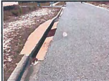
3. Photograph depicting an approximately 1 ft. X 2 ft. X 1.5 in. depression observed in the northbound travel lane near 302 Columbus Street. View to the south.
