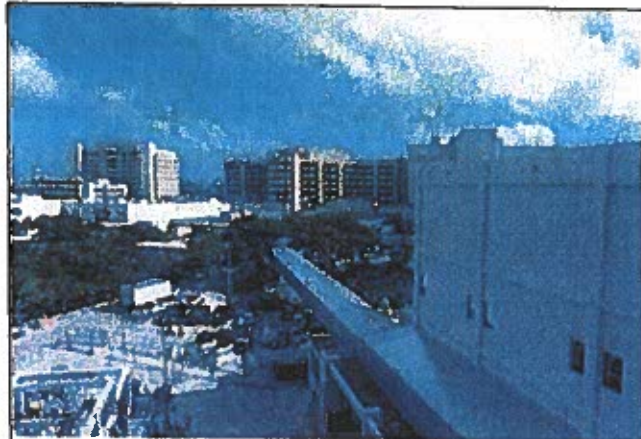
Mt. Sinai Medical Center Wind Retrofit Project 2005 Miami, FL
