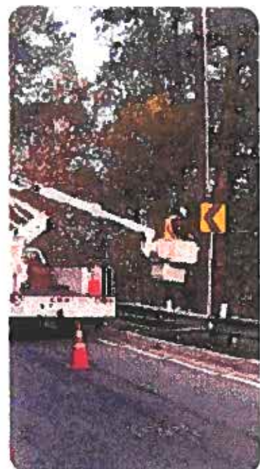
City Foot Traffic Street Electric & existing pole
