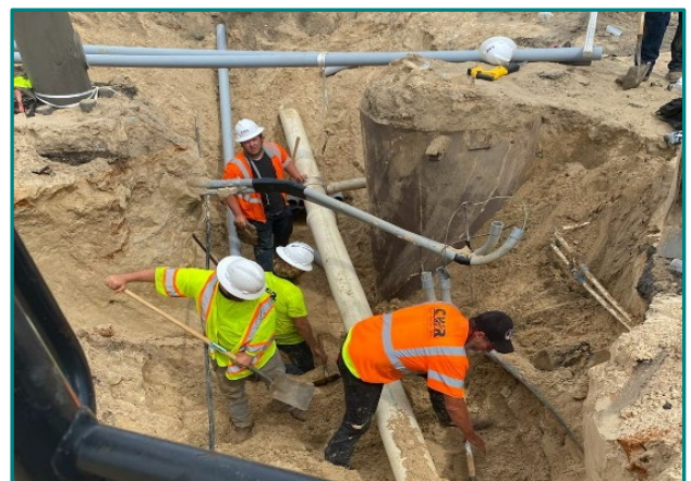
Installing new underground utilities and pipelines while working around existing infrastructure presents many challenges, requiring contractors to be cautious and diligent so no damage or disturbance occurs, while also ensuring no public services are interrupted.
