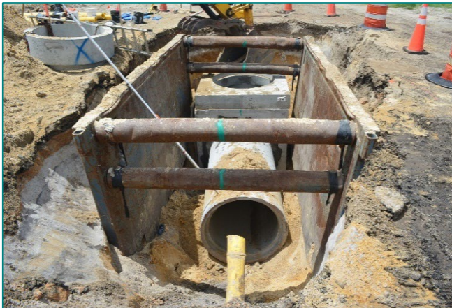
Installation of new 30" diameter storm sewer near San Vincente St. along Arnold Rd., moving north toward Back Beach Rd. The large steel box protects workers in the trench from cave-ins. Due to sandy, collapsible soils and multiple old utilities (gas line in foreground), progress is steady but cautious.
