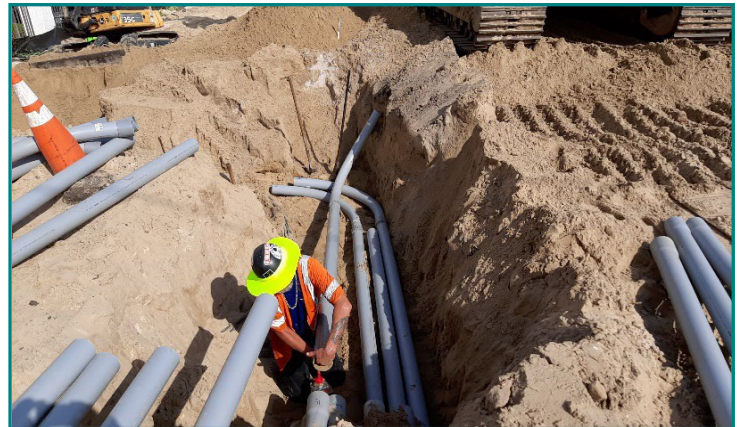
Crews work diligently and cautiously to lay piping to encase conduit lines critical to providing utility services to local residents and customers.
