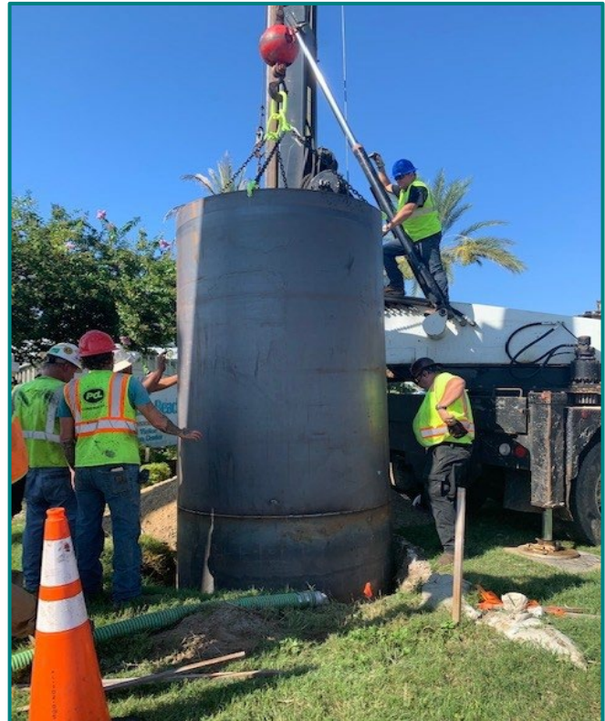
Ellis Crane Works completed drilled shaft construction for installation of new traffic signal mast arm pole in Segment 3.
