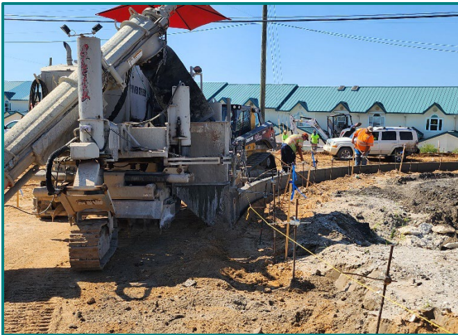
Crews recently started placing concrete for curb around the new roundabout at SR 79 & Front Beach Road.
