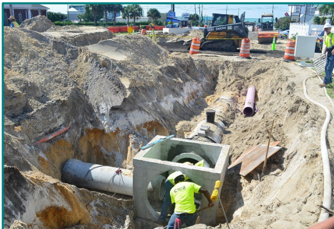
CW Roberts contractors work on installing a new storm sewer along Arnold Road south of Inca Avenue.
