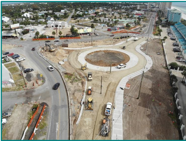
CW Roberts completed curb, road base course and sidewalk on portions of the new roundabout at SR 79 & Front Beach Road
