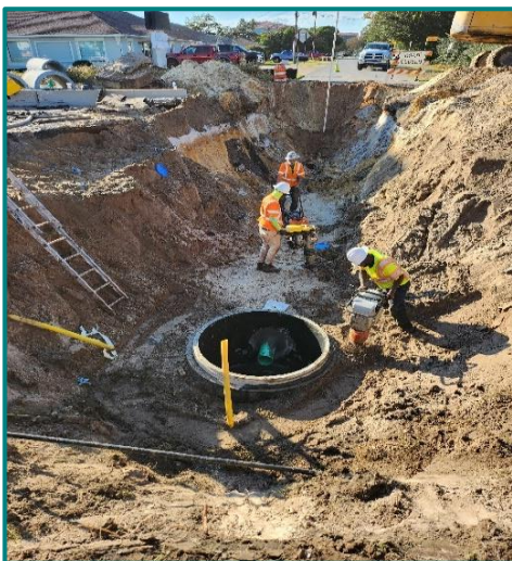
CW Roberts contractors work on compacting soil around the newly installed sewer manhole base along Arnold Road and Guava Ave.
