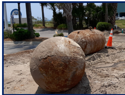
Utility coordination continues to be a challenge; propane tanks were found that had to be removed in the right of way by the Holiday Inn in mid-July.
