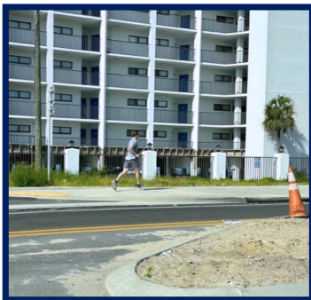
Jogger enjoying a beautiful morning on new sidewalks built to improve pedestrian safety by the roundabout on July 31, 2023.
