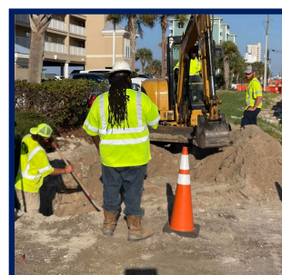
Crew is installing a new water main at Holiday Inn on Front Beach Road.
