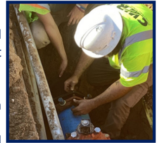
Crew setting a valve for the new water main on South Arnold Road.
