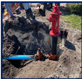
Crews installed a new fire hydrant which will be connected to the updated water main.
