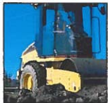
local company, MD Landscaping, assists with excavation and grading in Cochrane, AB
