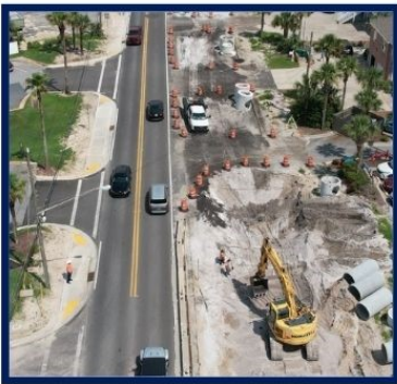
Continuing to install storm drainage infrastructure on the south side of Front Beach Road.
