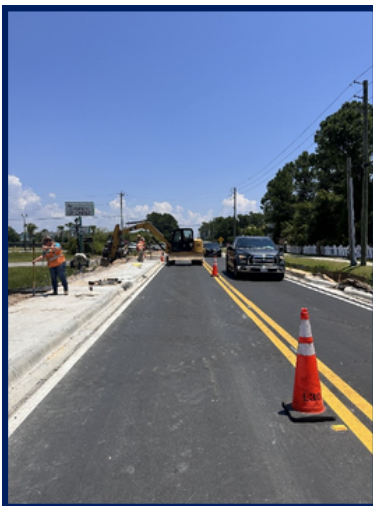
Grading the roadside swale in the area of The Church of Christ.
