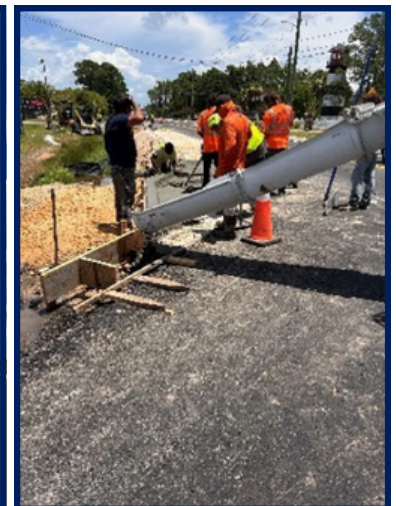
Constructing curb ramps on the west side across from Stone Harbor Apartments.
